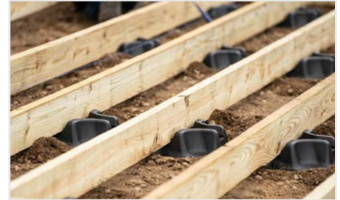
PLACE BLOCKS IN THE FIELD NO MORE THAN 5 FT. APART FROM EACH OTHER AND SO YOUR JOISTS ARE 16 IN. ON CENTER.
